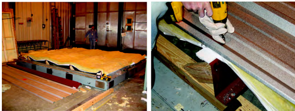
Figure 6 Installation of the fiberglass insulation and through-fastened steel-roof deck over the experimental roof.
